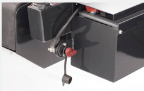
Battery master-switch for the rest period
