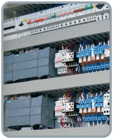
Electric board detail
