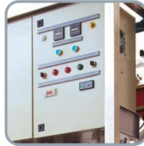
Electric board detail
